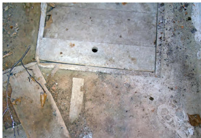
Access hatch to ventilation chamber in the floor
